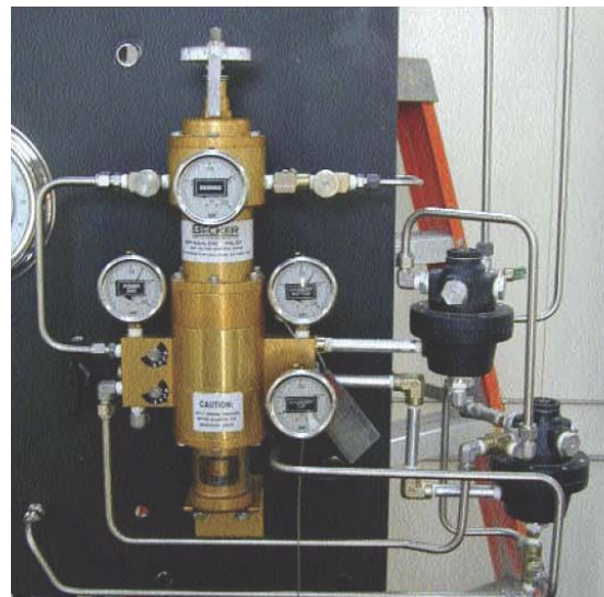
Figure 6 – A pair of Volume Boosters installed on a VRP-600-CH pilot feeding a large double-acting rotary piston actuator installed on a 30" ball type control valve to increase stroking speed. Note pilot is panel mounted.
